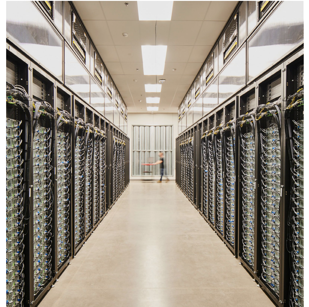
Apple's Reno data center, opened in 2012, takes advantage of the mild climate by cooling its servers with outside air whenever possible.
